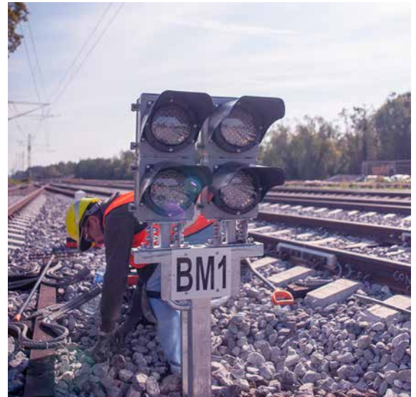
Mipro is renewing the signalling system on the Lääne-Harju track section in Estonia in cooperation with Estonian Railways Ltd.
