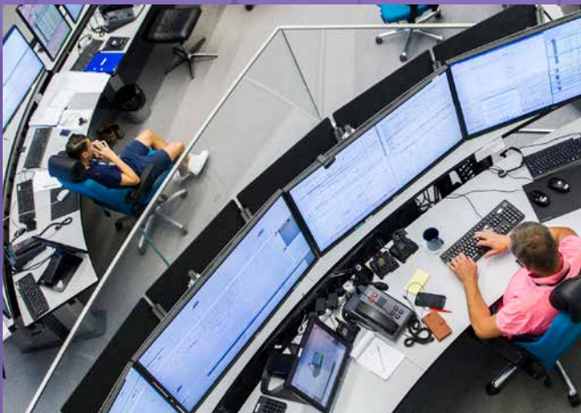
Mipro traffic management system manages Western Finland's remote control (TAKO) in the Viinikka traffic control centre of Fintraffic Railway Ltd.
